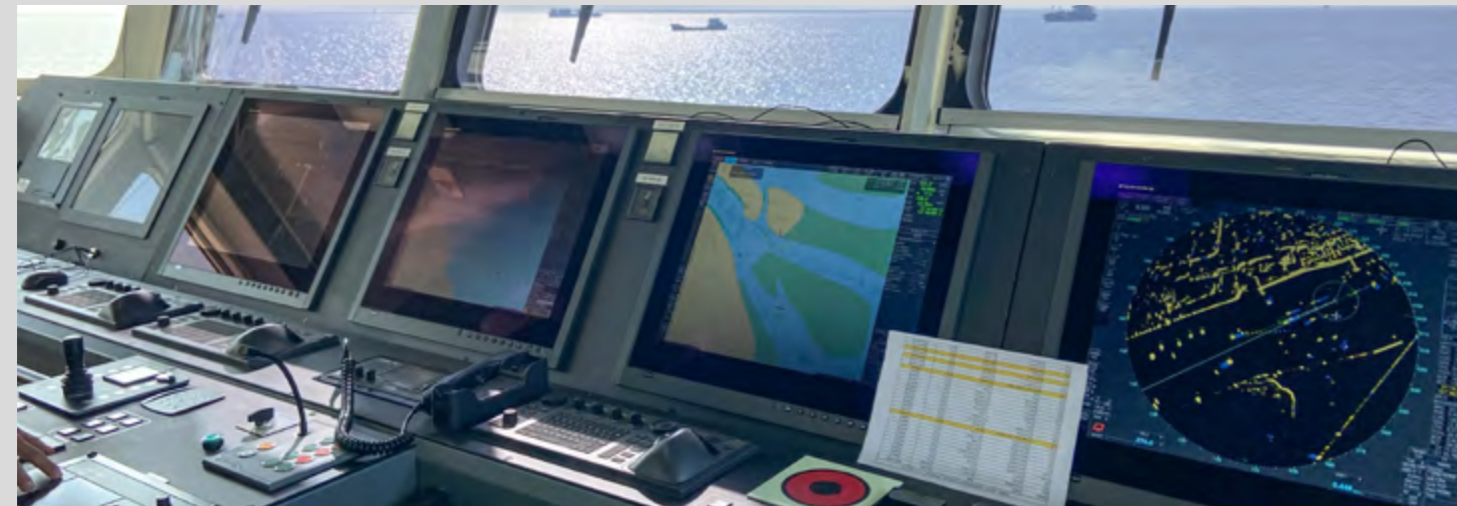
Navigation consoles for a Damen RoPax ferry
