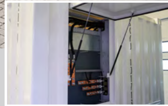
High voltage connection to containerized system
