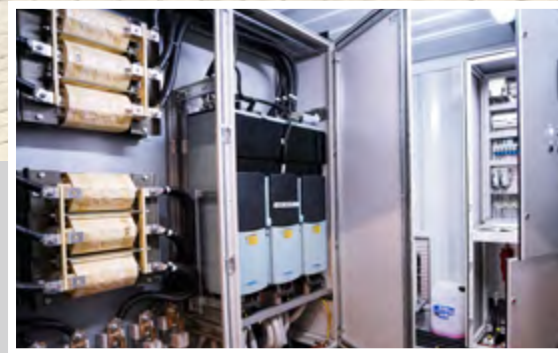
20ft containerized power system
