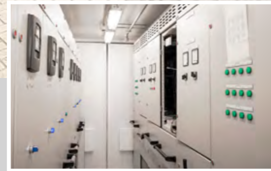
Power & control system intergrated in container
